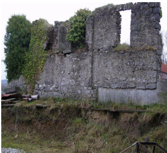
The last remaining wall
